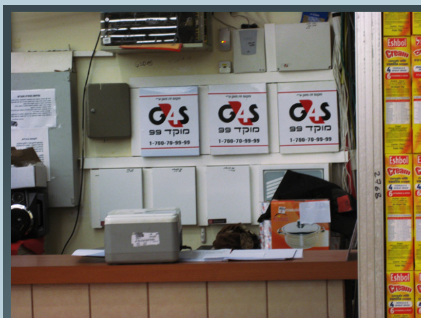
Systems of G4S installed in a supermarket in the West Bank settlement of Modi'in Illit. Photo: DanWatch
